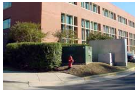
A street side hedge screens a transformer and other utilities from pedestrian view. The openly accessible side is oriented towards the least used pedestrian route.
