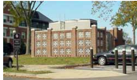
A decorative brick wall is used to screen a large pad of ground mounted mechanical equipment.
