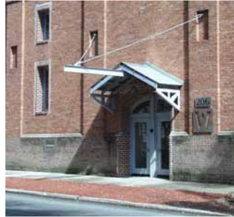
A new entry canopy provides weather protection while clearly differentiating itself as a modern addition to the old brick structure.
